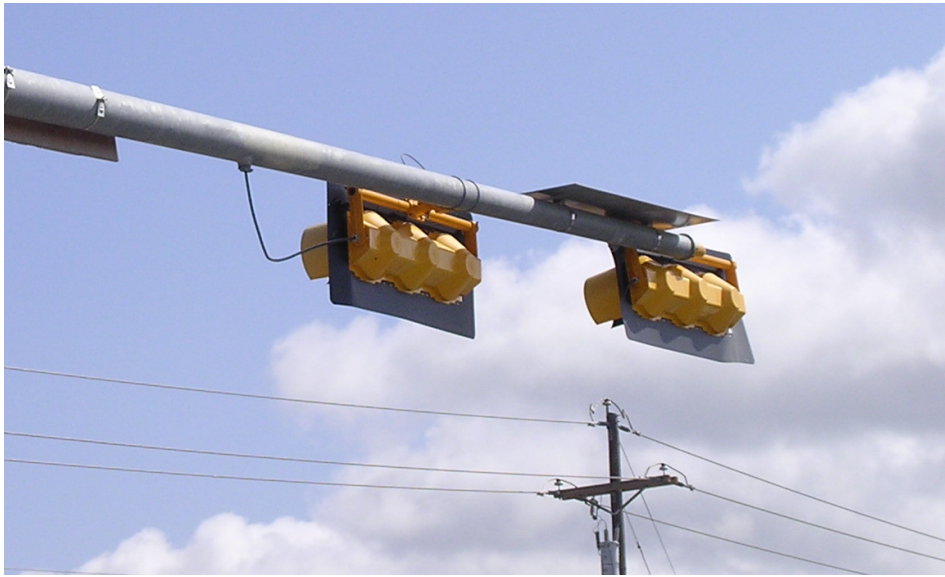
Figure 4.38: Traffic signals with squared-off backs attached to mast arm
