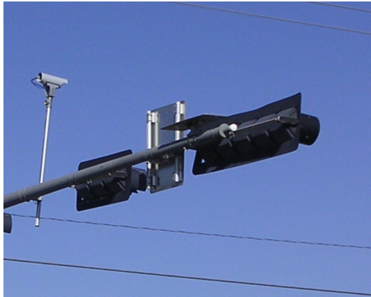
Figure 4.45: Traffic signals with V-shaped backs attached to mast arm
