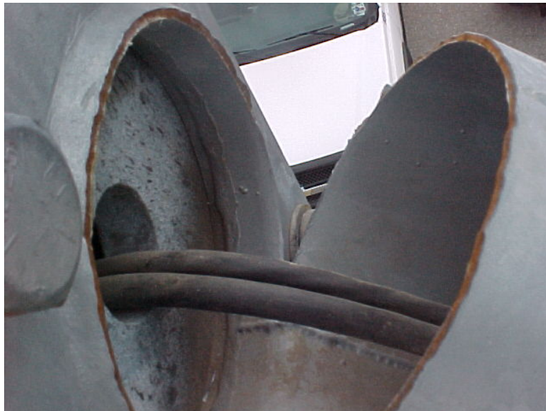
Figure 4.11: Rust is apparent in December 2003 fatigue failure
