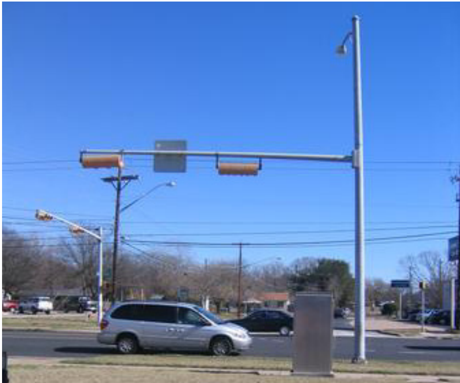
Figure 3.2: Traffic signal structure in Austin utilized for preliminary test setup
