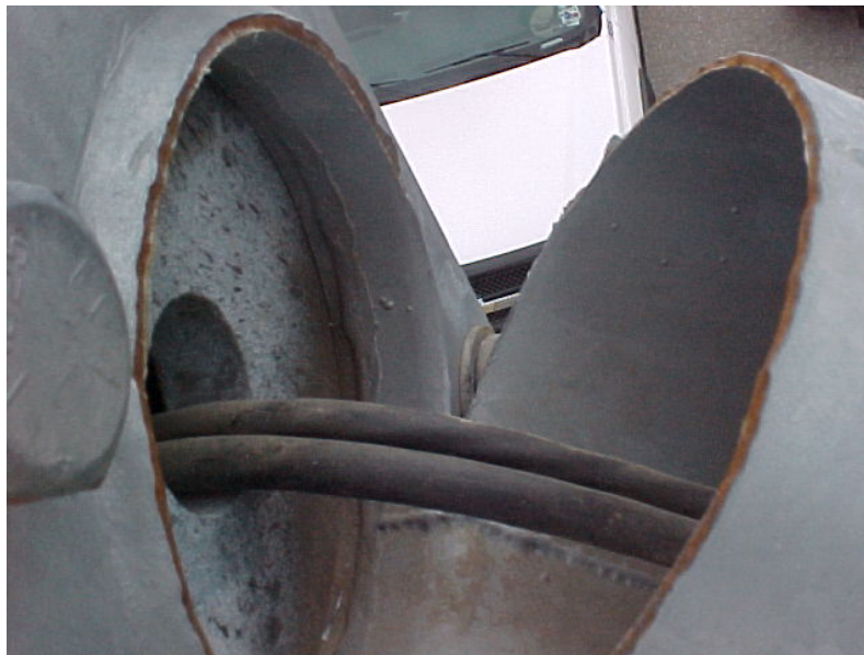
Figure 1.2: Failure due to fatigue crack initiated at top of mast arm
